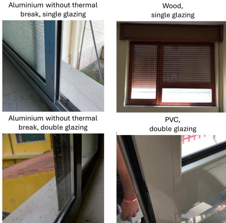
Figure 5. Example of typical transparent vertical components with different types of window frames and single or double glazing.
