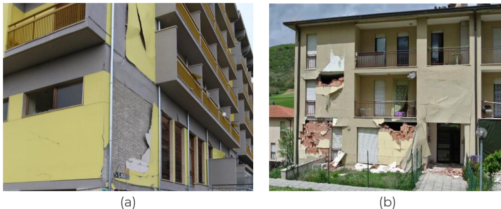
Figure 2. Example of observed damage to masonry infills and external thermal insulation (a: from Santarsiero et al., 2016; b: available online: http://www.reluis.it/images/stories/webinar-23-11-20/Prota-daPorto.pdf ).
