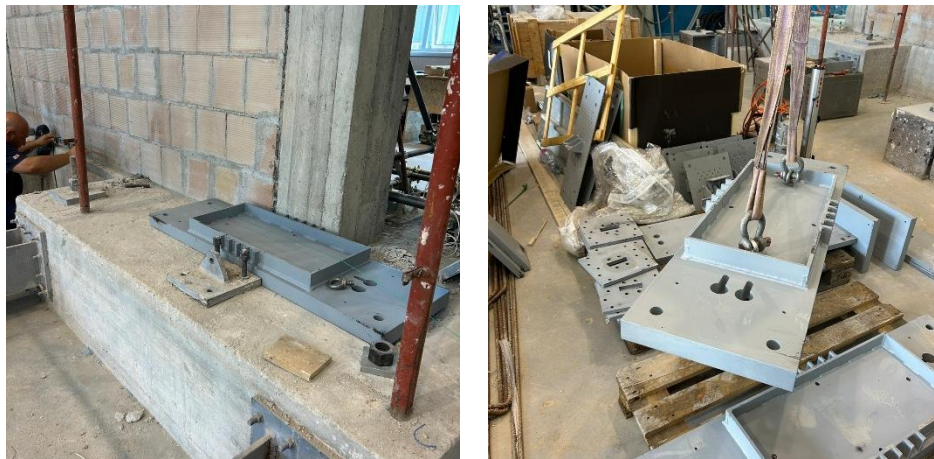
Figure 23. Example of a steel base plate realized for experimental tests as a part of the MULTICARE research project.
